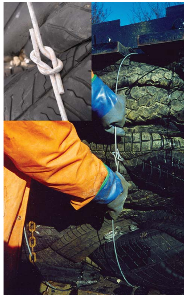
Figure 8 – Connecting the ends of the tie wires together (main picture) and after connection (inset)
