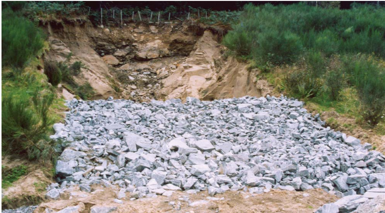
Figure D.9 – A gully eroded by the action of a debris flow
